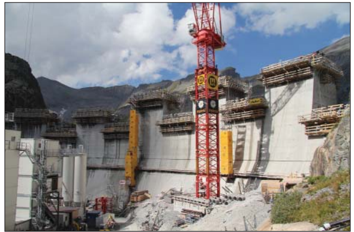
Obr. 13 Zariadenie staveniska pod päťou hrádze Vieux-Emosson, ktorej oporný múr sa navyšuje o 23 m Fig. 13 Site arrangement under the toe of the Vieux-Emosson dam, with the dam wall height being increased by 23m
