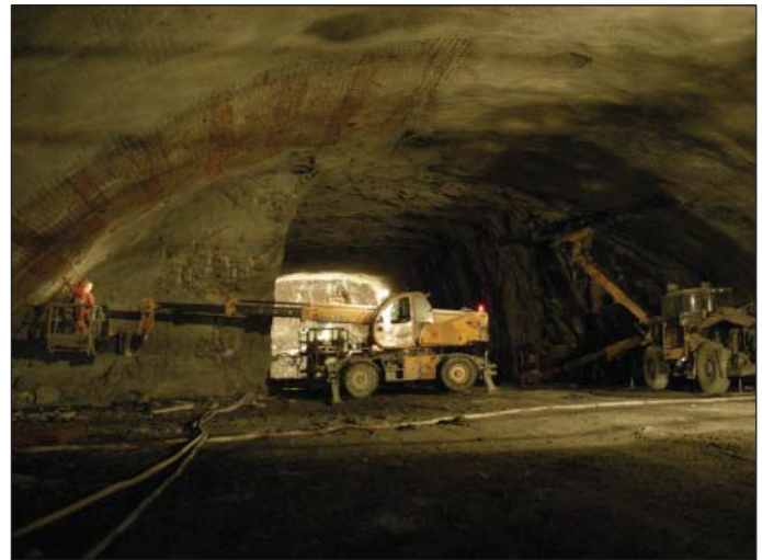
Obr. 11 Raziace a zaistovacie práce kaloty strojovej kaverne KMA Fig. 11 Excavation and installation of support in the KMA turbine hall cavern top heading
