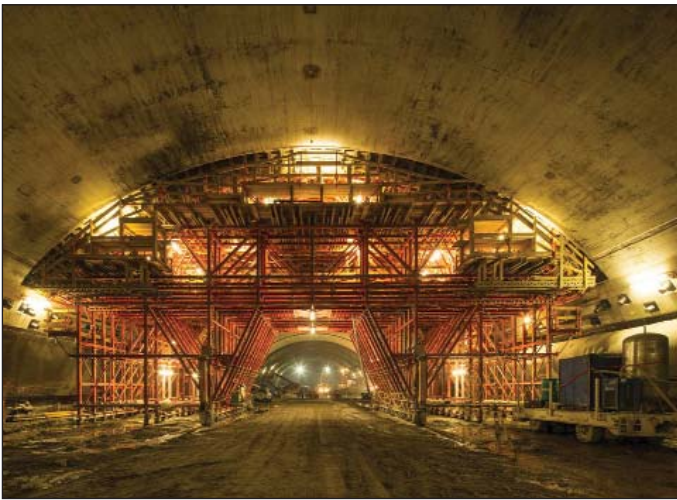
Obr. 12 Debnenie sekundárneho ostenia kaloty kaverny KMA Fig. 12 Formwork for the secondary lining of the KMA cavern top heading
